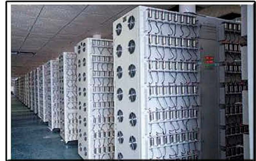
Cell Batching and Monitoring Stations
